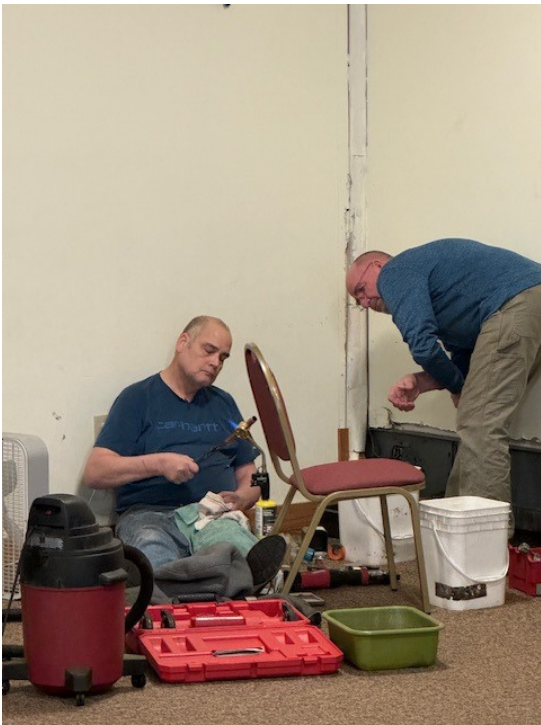
Jeff and Jessi fixing the leaky corner. This time it will hold.
